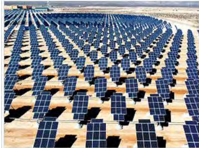
Nellis Solar Power Plant in the United States, one of the largest photovoltaic power plants in North America.
